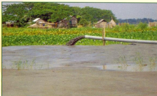
On going site and services plot development project at Shibchor, Madaripur (1st Phase)
